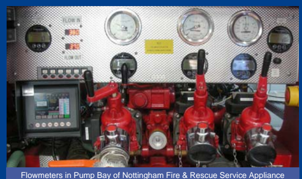
Flowmeters in Pump Bay of Nottingham Fire & Rescue Service Appliance
