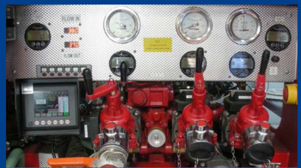
Flowmeters in Pump Bay of Nottingham Fire & Rescue Service Appliance
